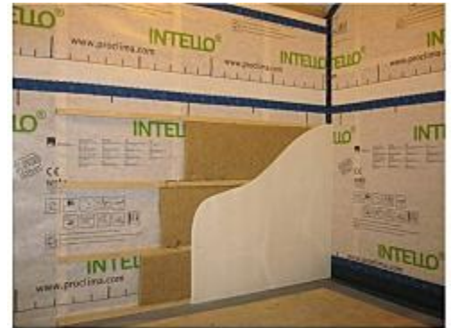
Airtight stud wall with service cavity (Airtightness Membrane fitted onto studs – No OSB Board)
